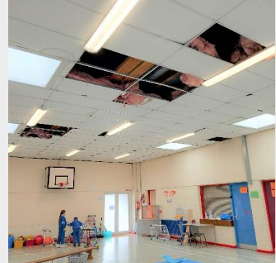
GP room with defective ceiling requiring substantial repairs.
