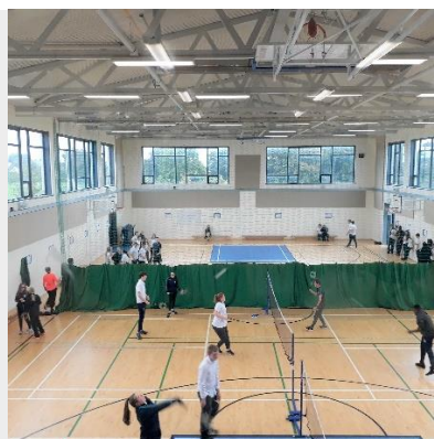
PE Hall high level windows maintenance requires health and safety measures.
