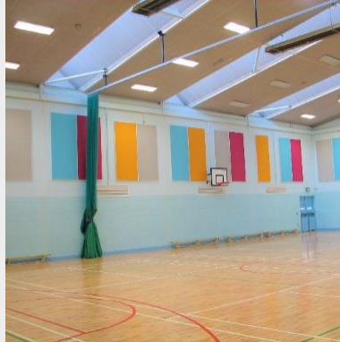
PE Hall after routine maintenance
